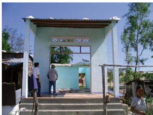
(a) A house collapsed in 2006 Typhoon Xangsane [54]
